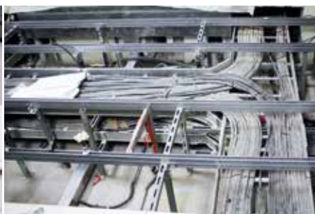
Fastening cable trays
